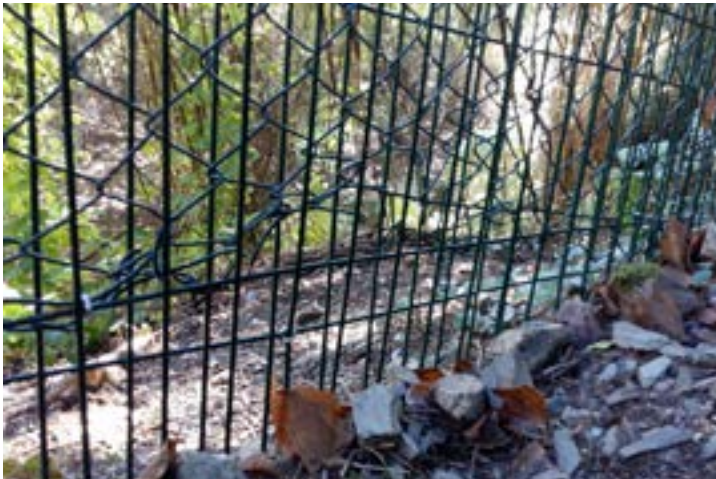
Figure 2.4. Repair of damage to chain-link fencing reinforced with electro-welded wire mesh suitable for wild boar.
