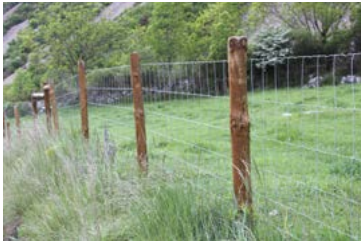
Figure 1.2. Fence made of knotted mesh with progressive density and wooden posts, suitable for rural settings. The mesh must also be buried in the soil to a depth of at least 20 cm.
