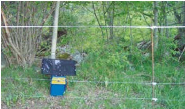
Figure 3.4. Power supply system with batteries and solar panels.
