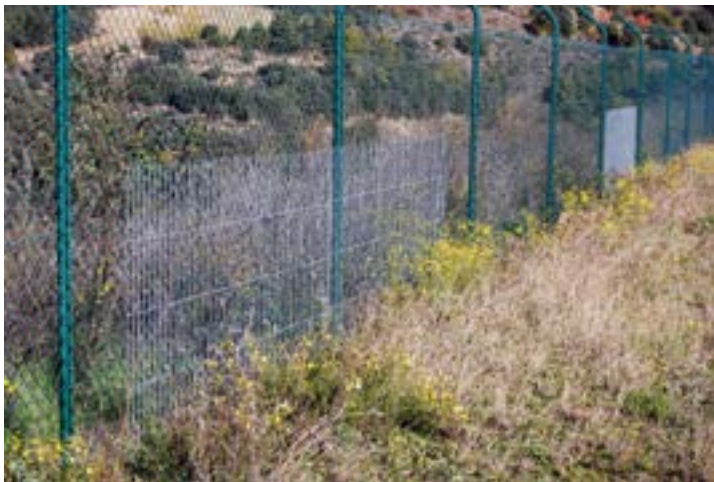
Figure 2.2. Reinforcement of chain-link fencing with electro-welded mesh installed along the bottom section.
