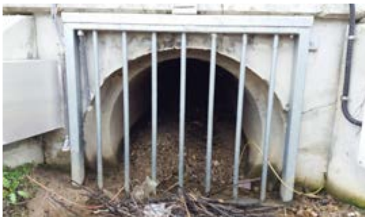
Figure 1.6. Protection of a drainage culvert to prevent wild boar from accessing an area enclosed by a perimeter fence.
